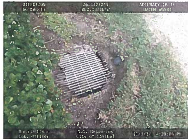
Figure 5 Discharge pipe of underdrain into stormwater catch basin at 4640 Rue Belle Mer.
